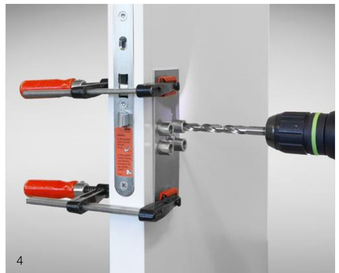
Image 4 Drilling from the righthand side of the door. Drill through the top righthand bushing on the drilling template. Important: do not drill into the lock case.
